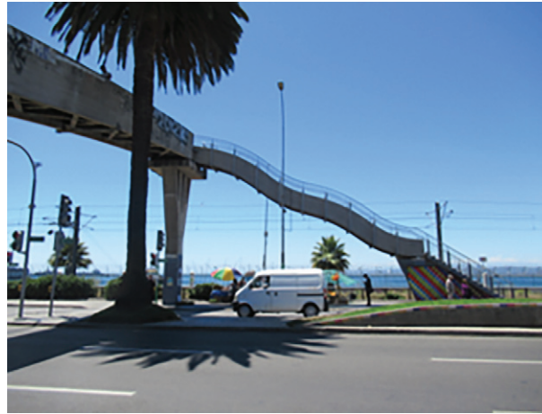
Figure 4 Severance aggravated by crossing facilities (footbridges) (Valparaiso, Chile).
